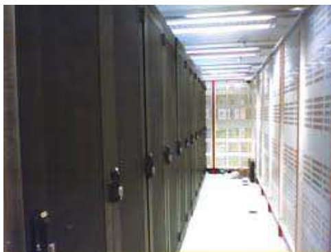
Fig. 10. Telephone equipment rack.
