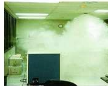
Fig. 11. Total flooding gaseous system in action.
