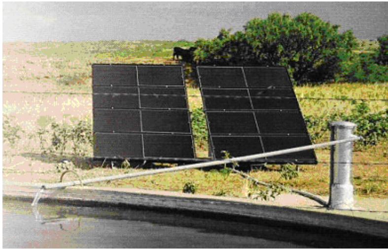
Fig. 3. Solar pump for recycle waste water from the down stream to upstream storage reservoir
