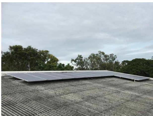
Fig. 4. 4.2 kW solar PV grid-connected in AIT
