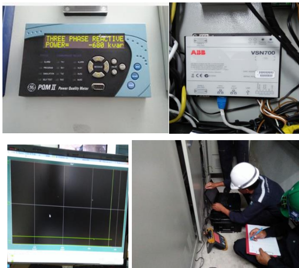
Fig. 3 Electrical measuring instrument and ABB monitoring and communications.
