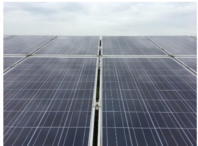
(a) PV panel surface and installation array
