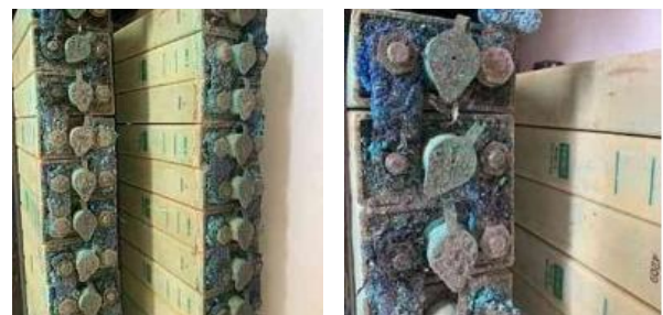
Fig. 11. Oxide on junction of Battery Backup.
