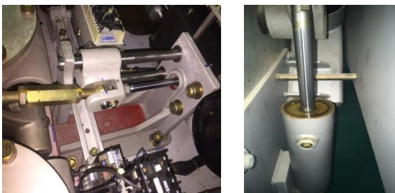
(a) Hydraulic pump leakage (b) CB damper leakage
