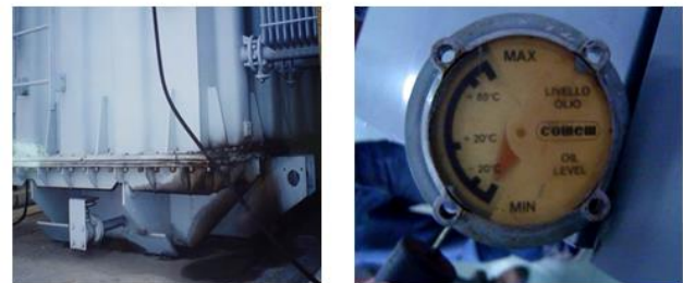
(a) Oil Leakage (b) Oil Level Gauge Defective
