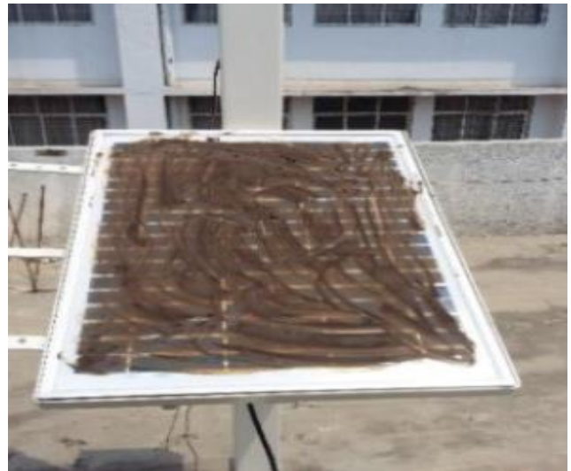
Fig. 11. Mud applied on solar panel.
