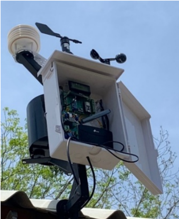
Fig. 2. Part of automatic control systems and network display.
